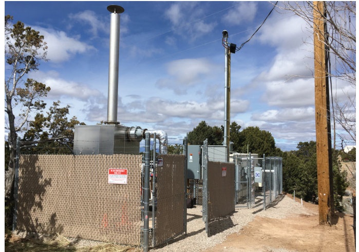
DBS&A creatively engineered larger SVE equipment to fit within a space that is shared by highway ROW and a utility corridor.
