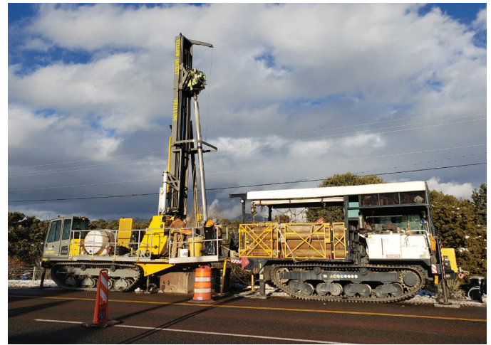
DBS&A provided oversight and CQA for the installation of 20 wells, most of which were installed in highway ROW.
