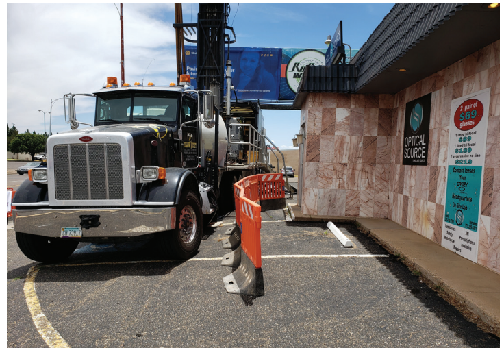
The drill rig was parked seven feet from the front door of a small business to facilitate installation of a critical remediation well.
