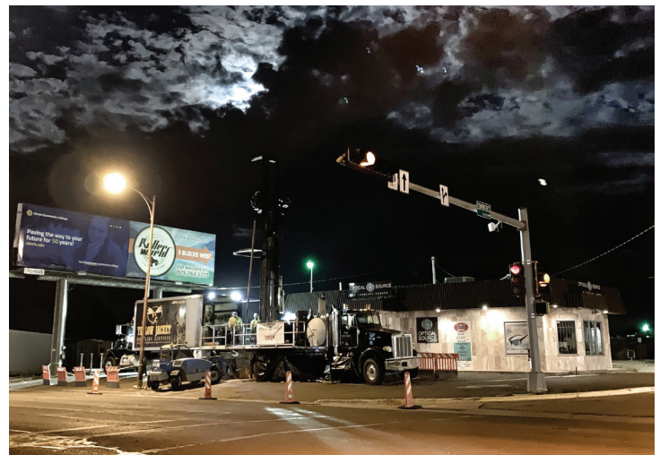
Overnight drilling was employed to expedite drilling activities in extremely close proximity to a small business.
