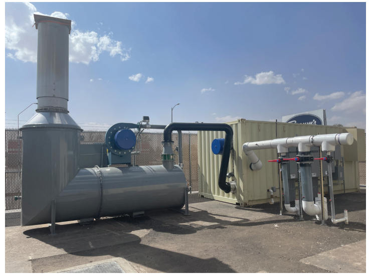
Remediation components include a 1,000-cfm thermal oxidizer and modular vapor extraction and groundwater treatment equipment.
