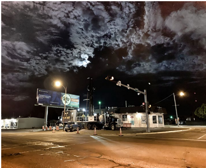
Overnight drilling was employed to expedite drilling activities in extremely close proximity to a small business
