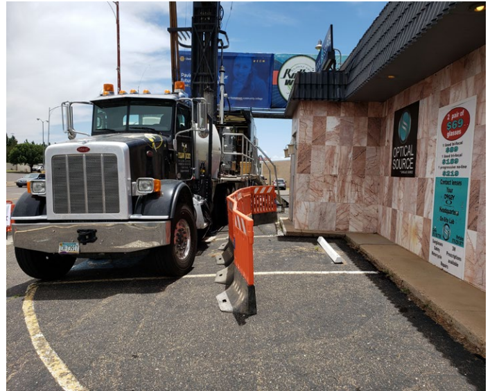
The drill rig was parked 7 feet from the front door of a small business to facilitate installation of a critical remediation well
