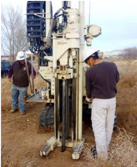
Rapid direct-push drilling methods used for soil vapor testing at a closed landfill.
