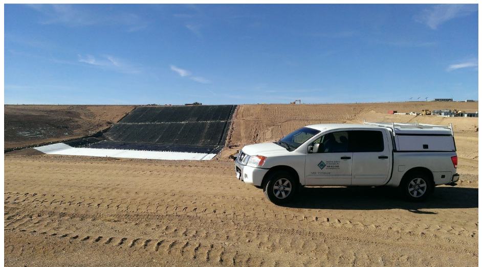
View of GCL and HDPE liner installation progress during recent Construction Quality Assurance project.
