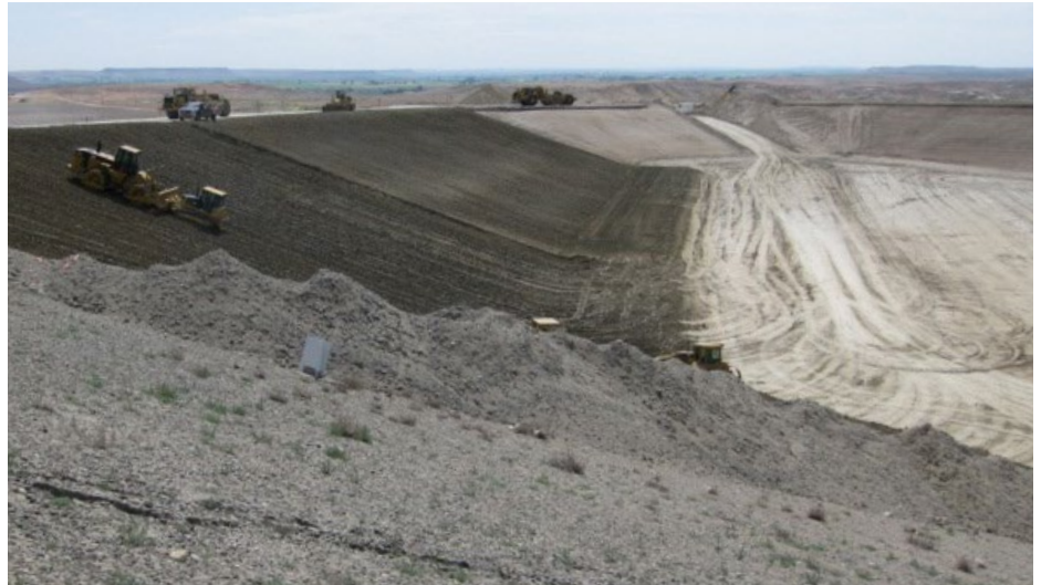
DBS&A obtained regulatory approval an alternative earthen cover system for two hazardous waste disposal trenches.
